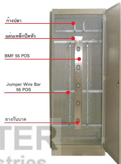
Detail of BMF Set and Jumper Wire Mount on Floor Mount Cabinet
